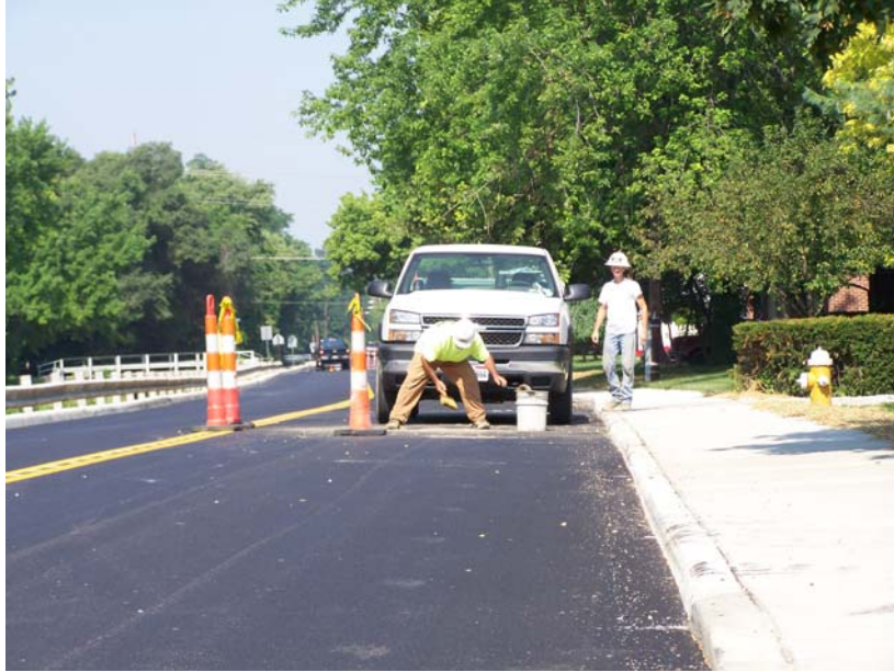
From left, Dwayne Heidel and Charles Kindrick of Dixie Excavating finish working on the asphalt around the manhole covers on Gibbon Road.
